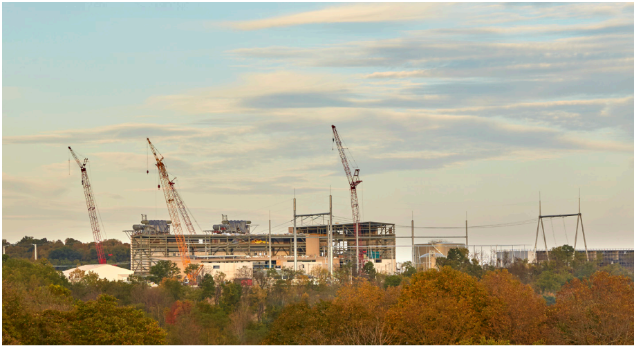
Construction progresses at the Tenaska Westmoreland Generating Station site near Smithton in South Huntingdon Township, Westmoreland County.
